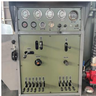
操作阀面板 Operating valve panel
