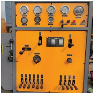
操作阀面板 Operating valve panel
