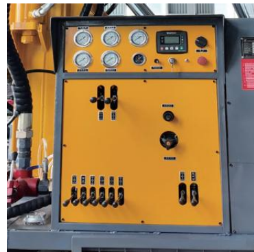
操作阀面板 Operating valve panel
