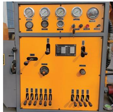
操作阀面板 Operating valve panel
