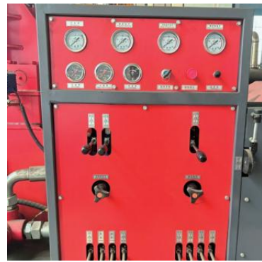
操作阀面板 Operating valve panel
